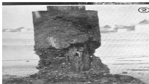
Fig. 1 Deterioration of concrete cover
