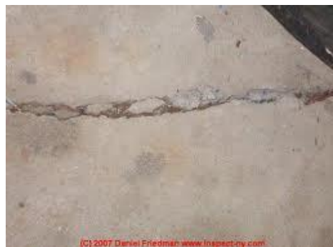
Fig.1 Cracks due to Early Frost Damage
