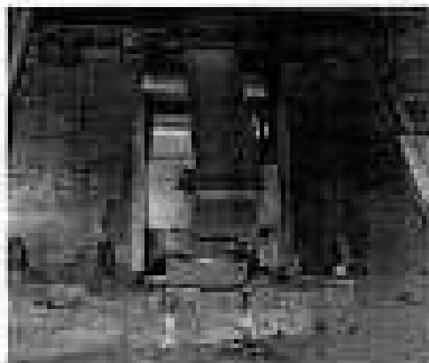
Fig 3.1.2 Shows the furnace with pre heating properties
