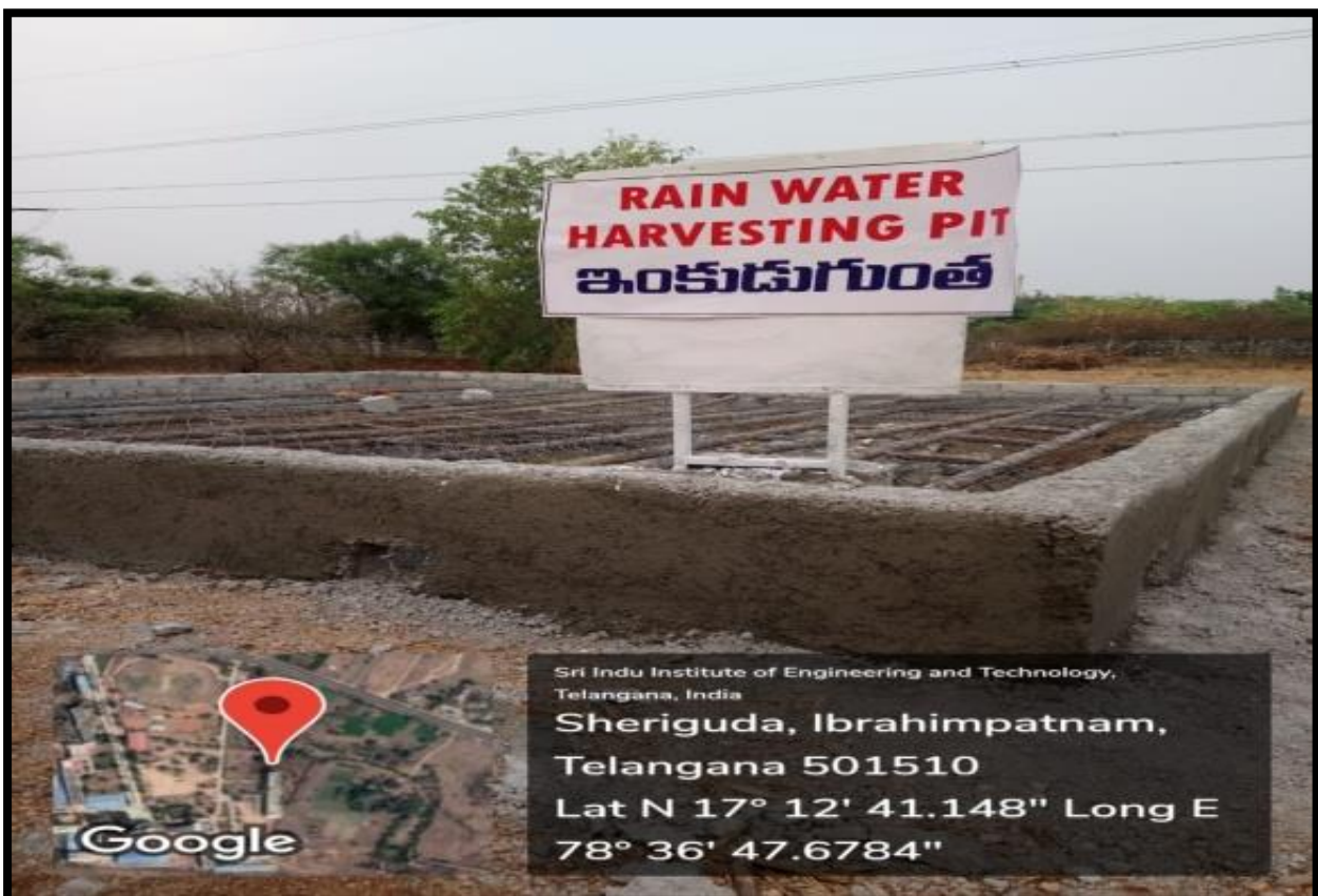
Rain Water Harvesting Pit
