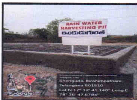
Rain Water Harvesting Pit
