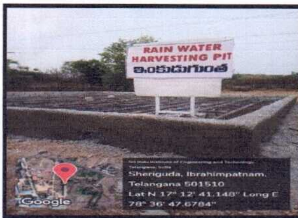
Rain Water Harvesting Pit
