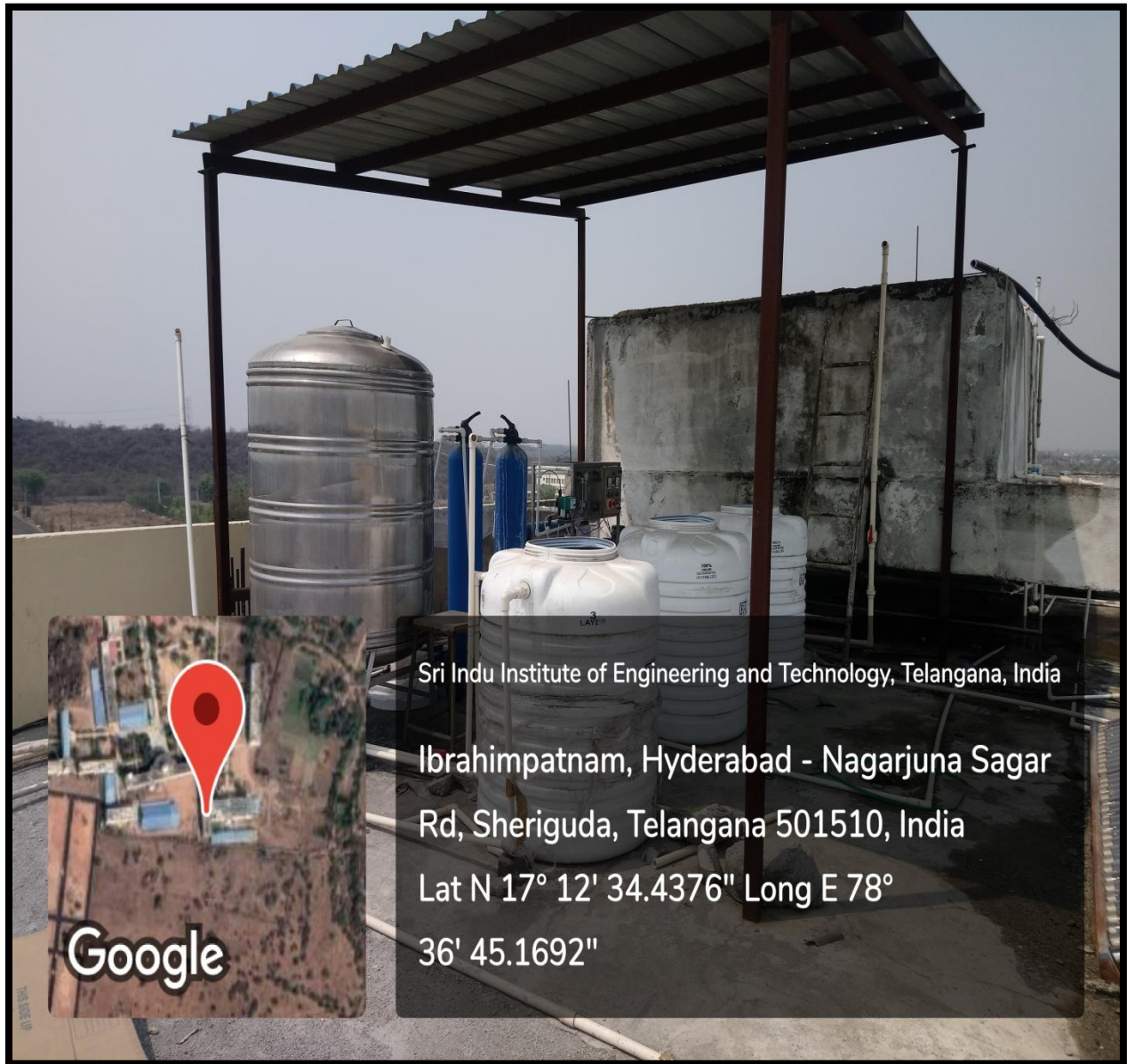
RO plant with storage tanks
