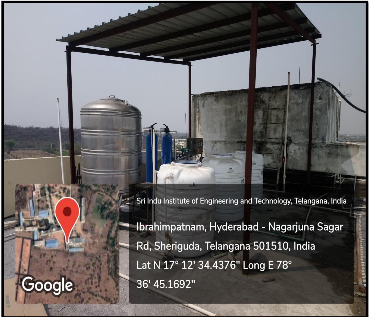
RO plant with storage tanks
