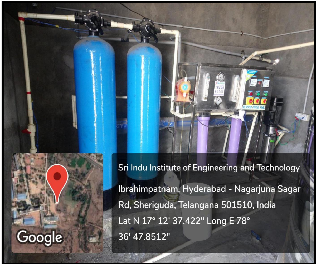
Recycling waste water through RO Plant
