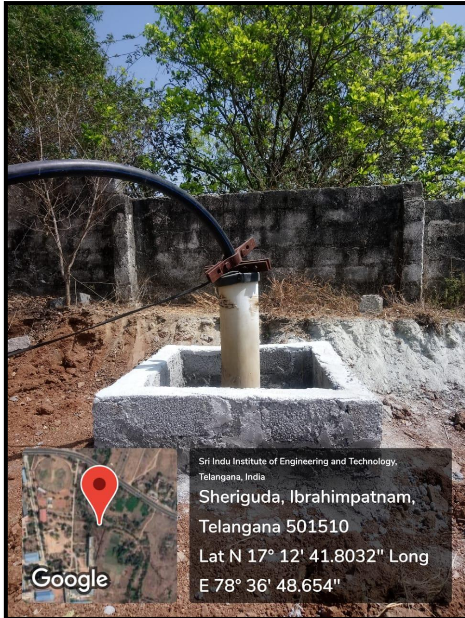
Borewell with recharge pit
