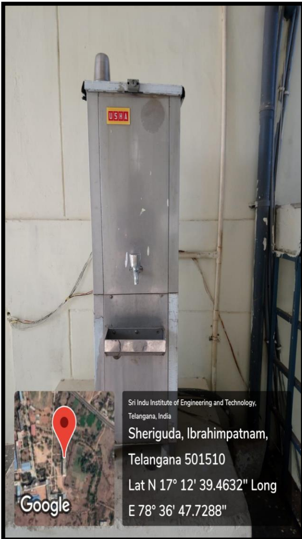
Drinking water Cooler
