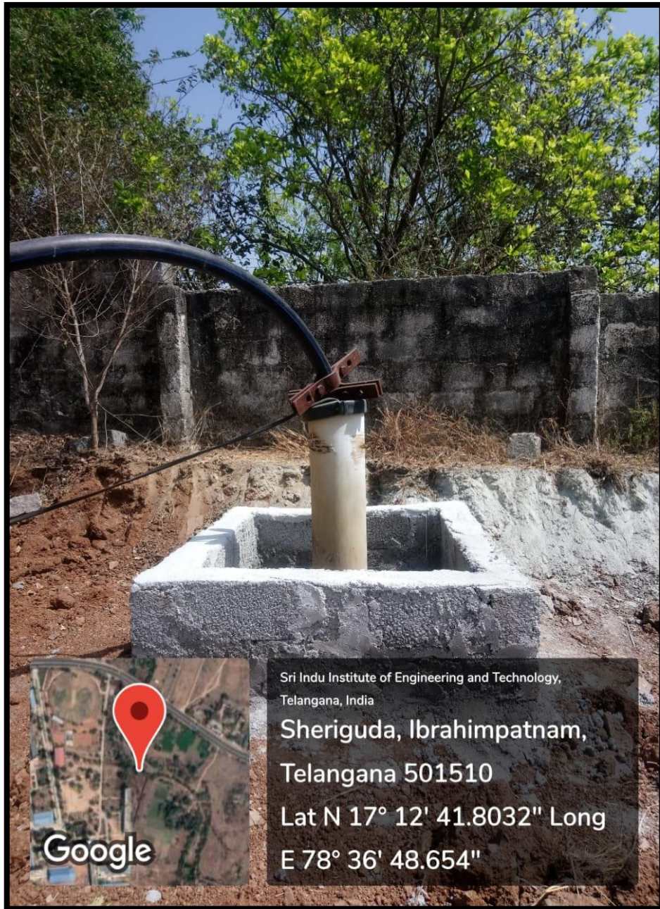
Borewell with recharge pit
