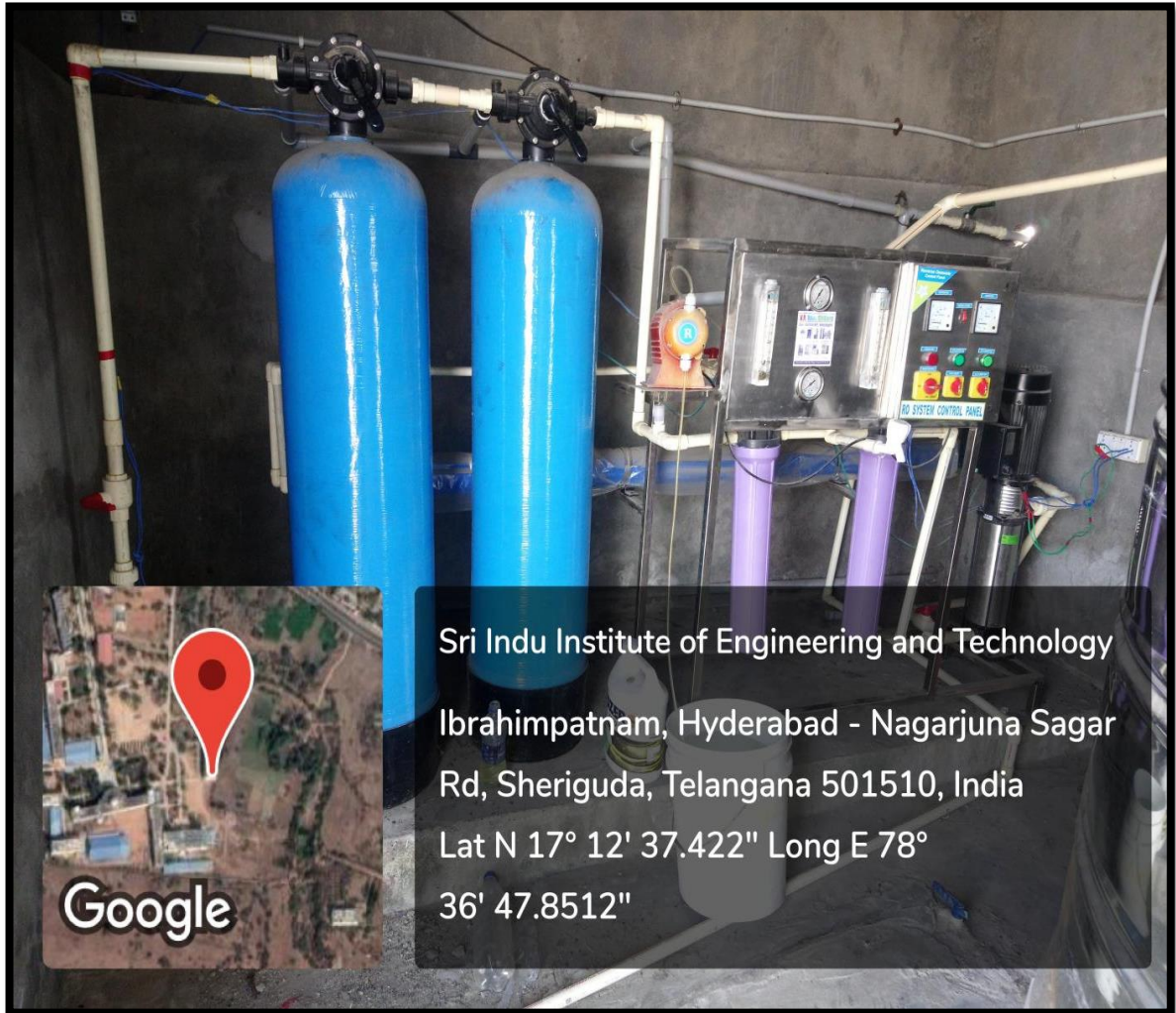
Recycling waste water through RO Plant
