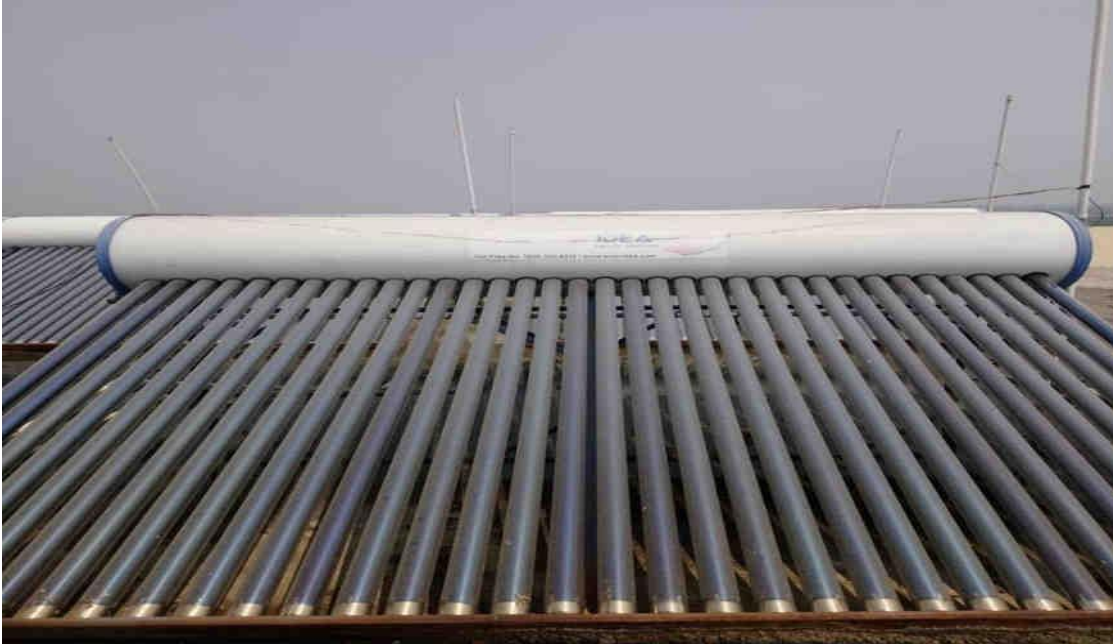
Solar water heater
