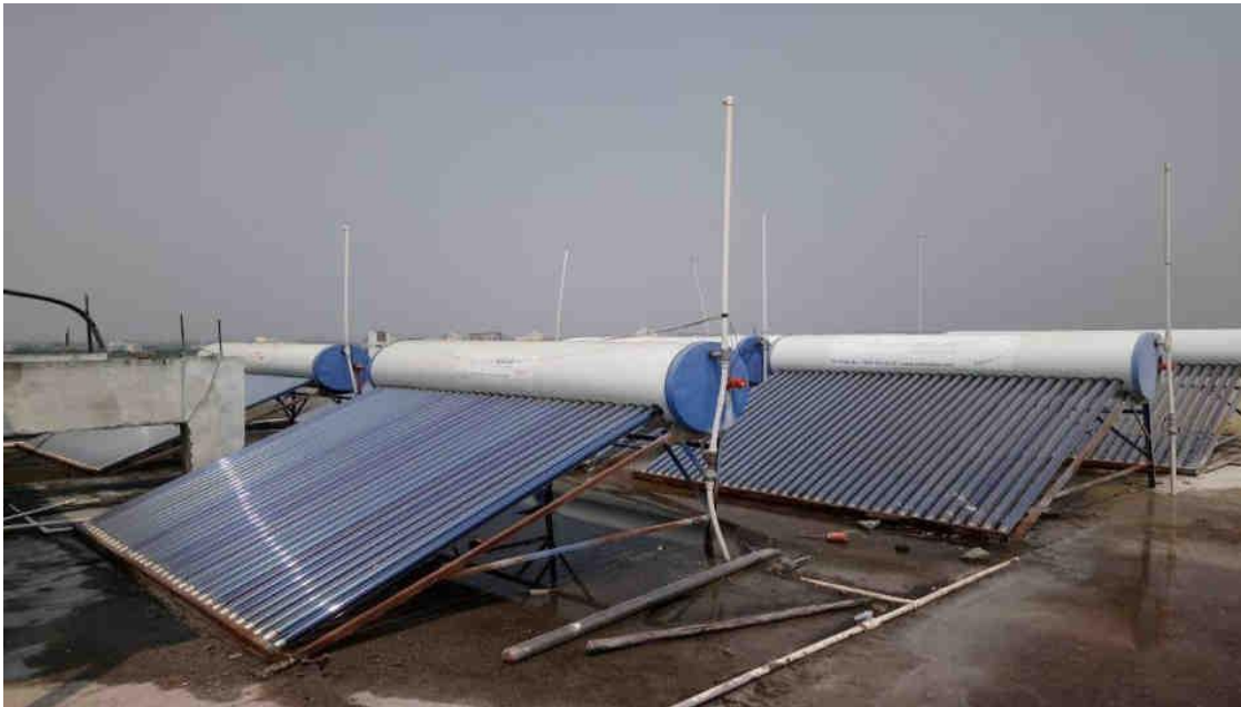
Array of solar panels installed on rooftop of college hostel building.
