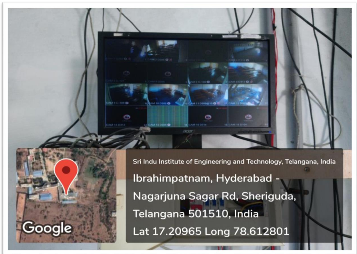
Surveillance CCTV monitoring
