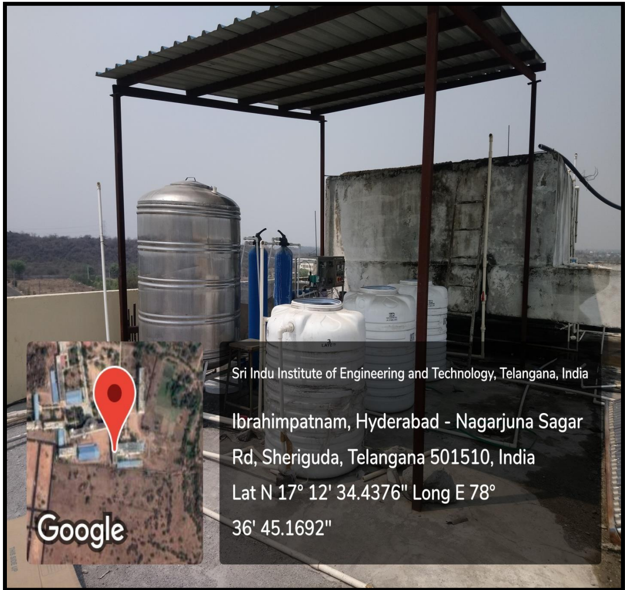
RO plant with storage tanks
